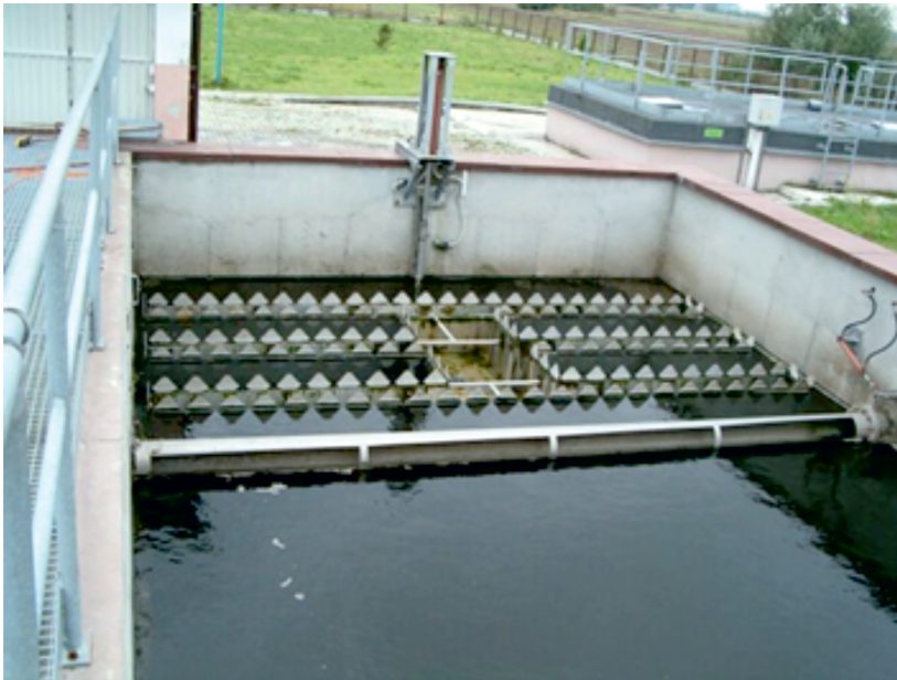
Fig. 17. Outlet from a rectangular settler with three double-sided weir channels and scum trough
