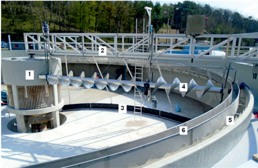
Fig. 21. Empty horizontal-flow sedimentation tank in Gorzów Wielkopolski (Poland) with central distribution chamber (1), rotating bridge (2), sludge scraper (3), scum removal screw (4), peripheral weir channel (5), and scum baffle (6)
