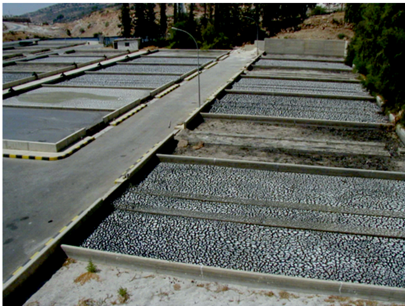
Fig. 54. Sludge drying beds at a small wastewater treatment plant (Ethics Infinity Pvt. Ltd.)
