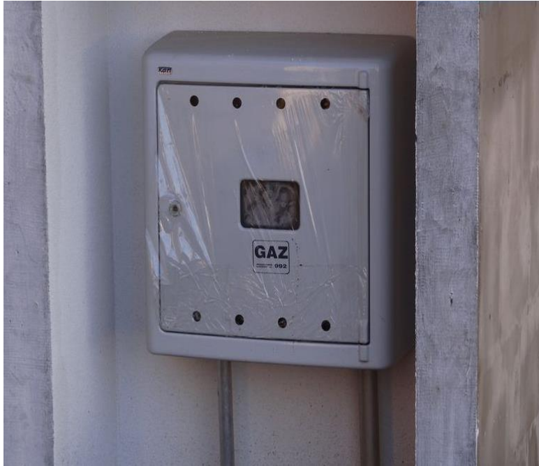
Gas box for one gas meter
